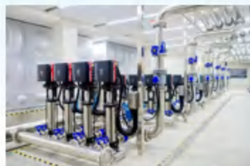
Water Treatment Equipment
