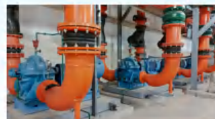
Secondary Water Supply Pumping Station Monitoring Platform
