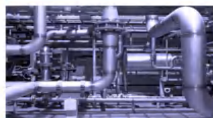
Pipe Network and Utility Tunnel Monitoring Platform
