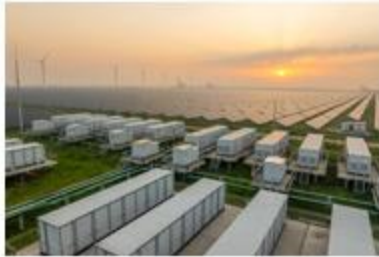
Energy Storage EMS
