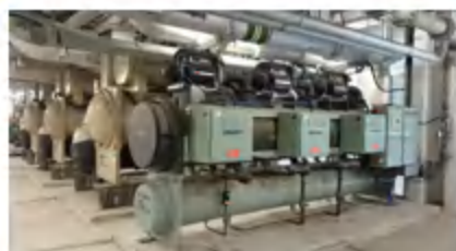
Smart Cooling Monitoring Platform
