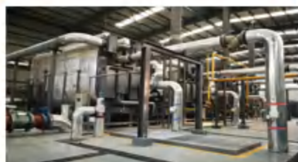
Smart Heating Monitoring Platform
